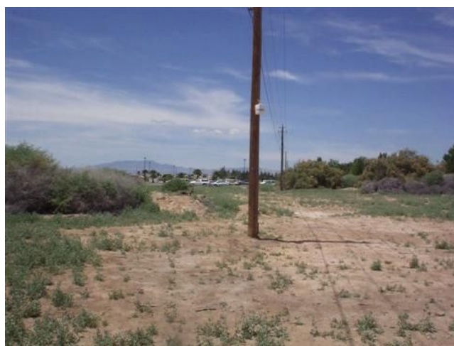
Figure 3-3. Sampler Mounting on a Utility Pole
